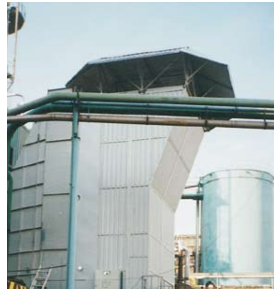
CamPulse Filter System for GE Frame 6 unit in Spain.
